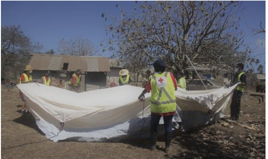
Red Cross teams set up a temporary shelter in the village of Kanokupolu, western Tongatapu, on Friday 21.
