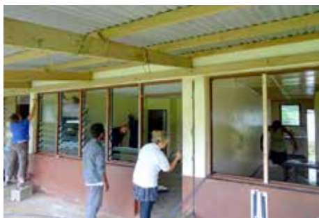
The team hard at work repairing and replacing louvres on each unit.
