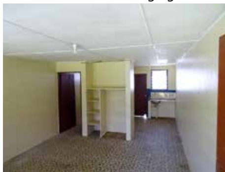
The inside of one unit painted, cleaned, fixed and awaiting new tiling in the kitchen.
