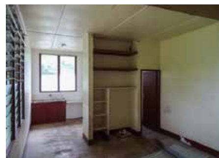
Before the work began: a family will live in this typical two room unit, with a bathroom, kitchen and lounge room-cum-bedroom.
